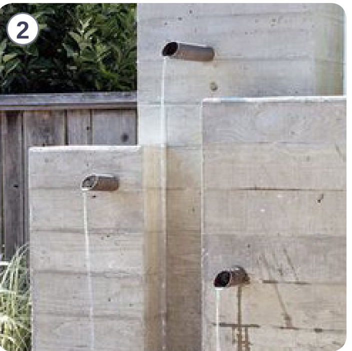
Pipes to direct roof rainwater into swale
